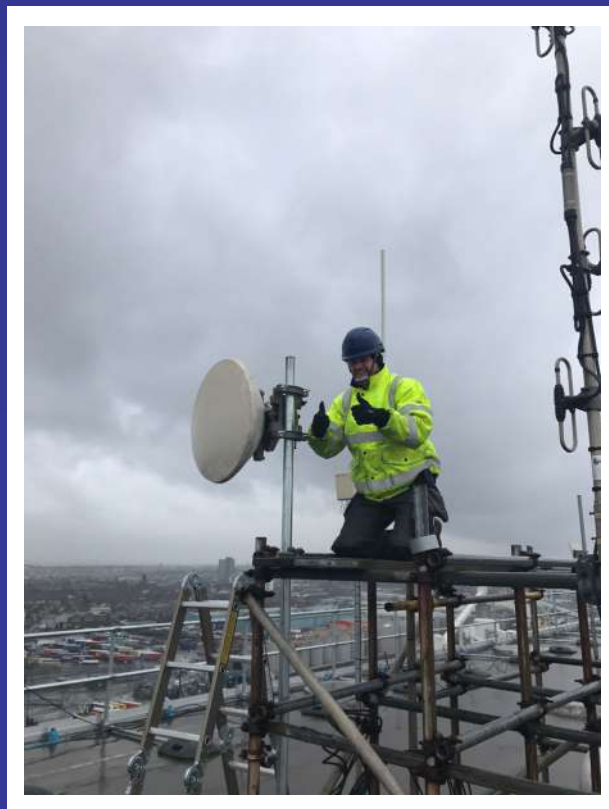
Fig 2. Ensign engineer, Patrick Murray, braves the weather during the Siklu link installation.
